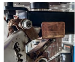
Built-in grounding point
